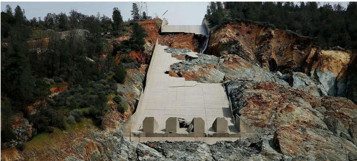
Photograph: Oroville Dam Spillway Failure. Santiago Mejia / The Chronicle
